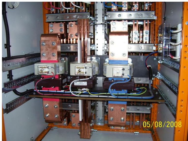
Bus bar and CT assembly for the Weipa Health Care Facility new Main Switchboard
